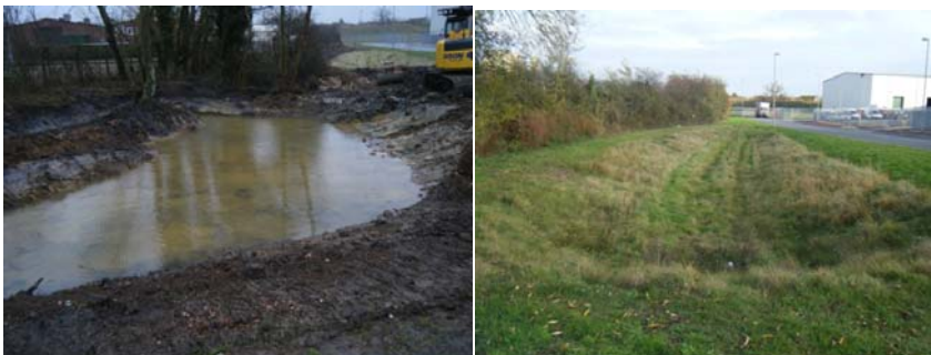
New developments and drainage schemes in Wiltshire have provided opportunities to introduce ponds and swales to improve water quality and habitat
