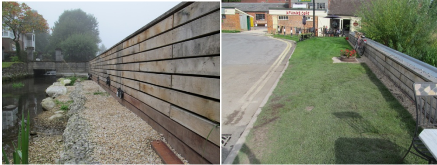
At Marlborough a flood alleviation scheme was jointly funded by the Environment Agency, Wiltshire Council and Marlborough Town Council.
